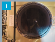
h i Air scrubber with spray tower.
