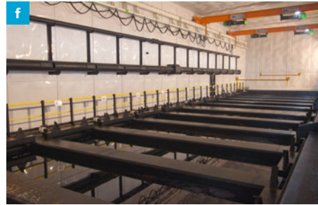
The pre-treatment line seen from the inside with polyethylene enclosure.
